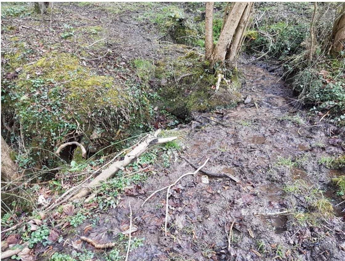
Saturated made ground/seepage
