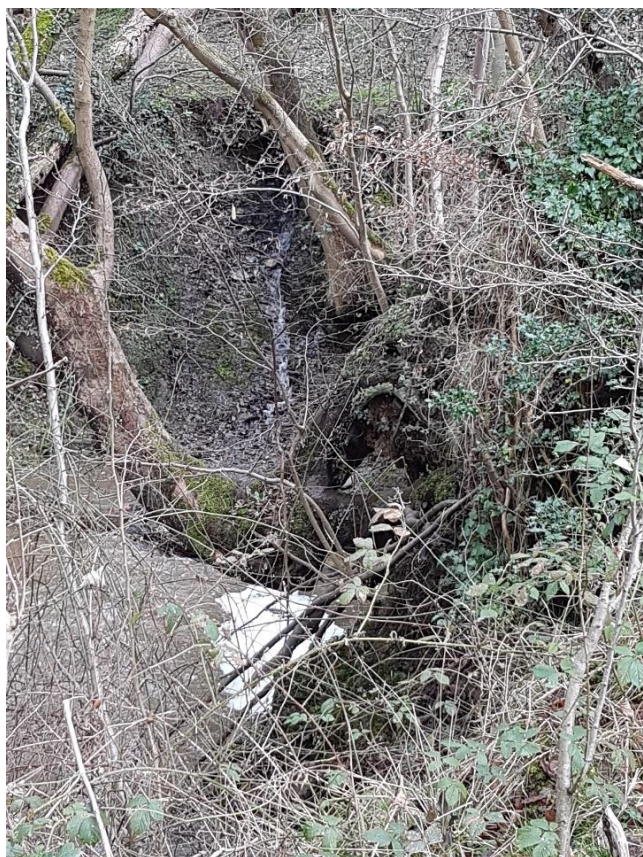
Seepage through made ground creating small waterfall
