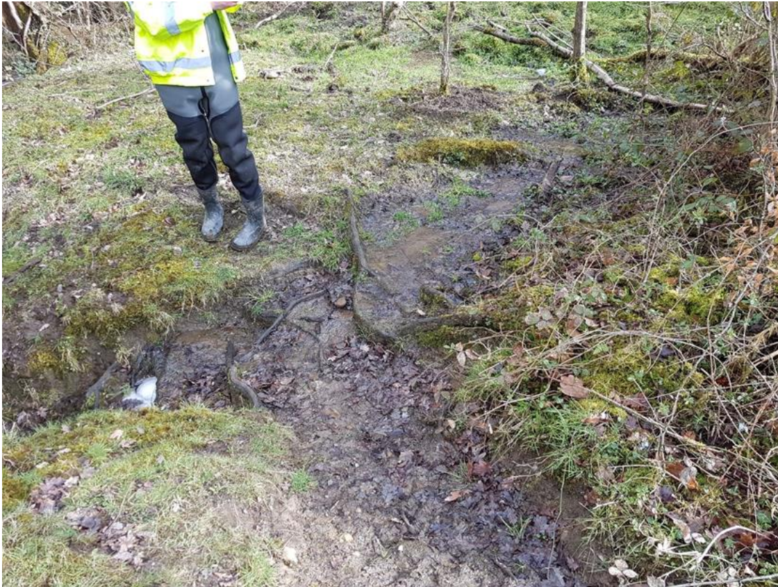
Saturated made ground/seepage
